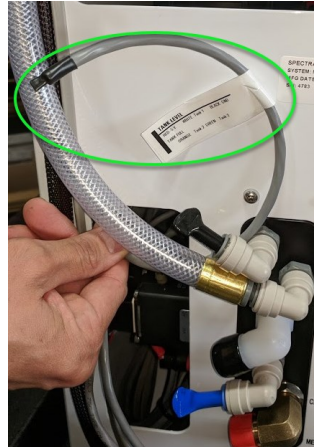
5 Conductor wire: Tank Full Switch, Green + Orange
