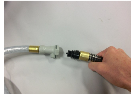
Attaching intake service hose to the hose connecting to the sea strainer.
